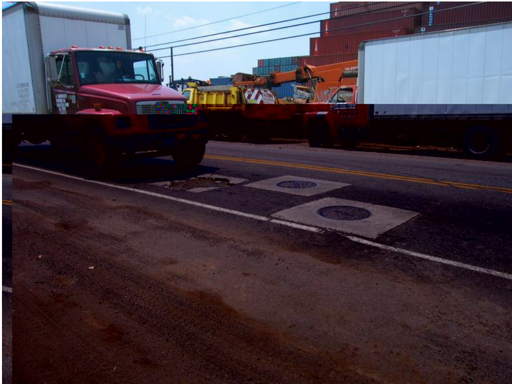
Figure 2. Locating manufactured BMPs in the roadway is sometimes an only alternative. It is essential, however, that traffic can be directed around the facility while it is being maintained. If possible, designers are urged to find a location that provides relatively easy access. (Photo courtesy of Dr. Qizhong (George) Guo, Rutgers University)
