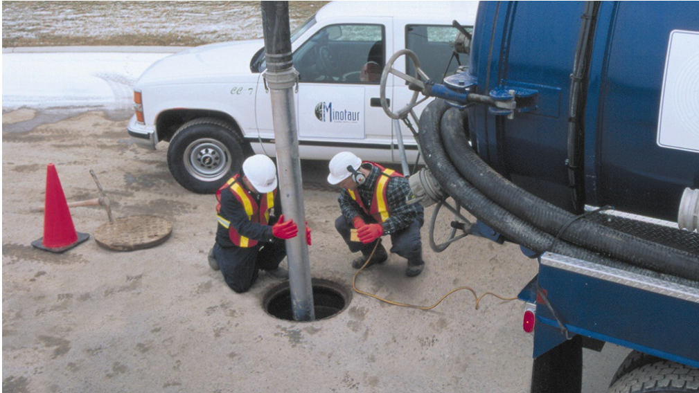
Figure 3. All personnel who conduct maintenance on manufactured BMPs should have completed confined space training. (Photo courtesy of Scott Perry, Imbrium)
